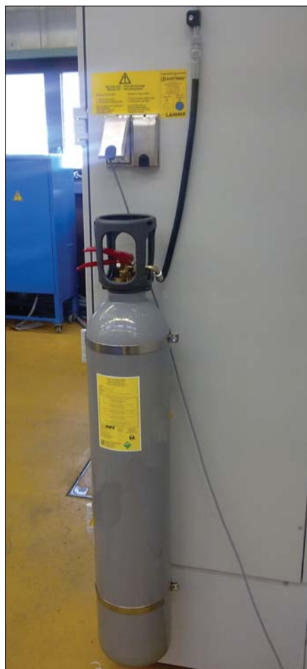
Typical manually activated fire system
